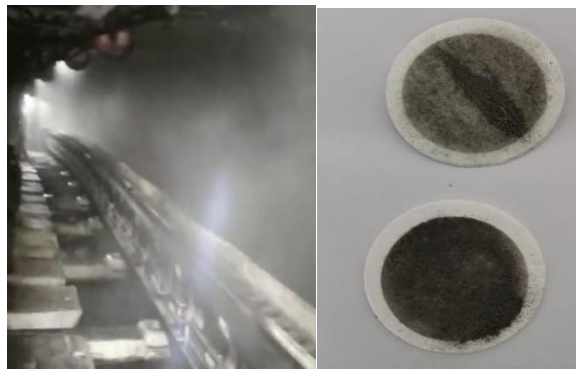
Fig 1. Dust pollution on site
